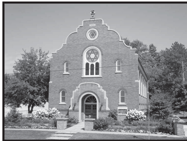
Restoration work was done to maintain the original style of the building, built in 1928.
